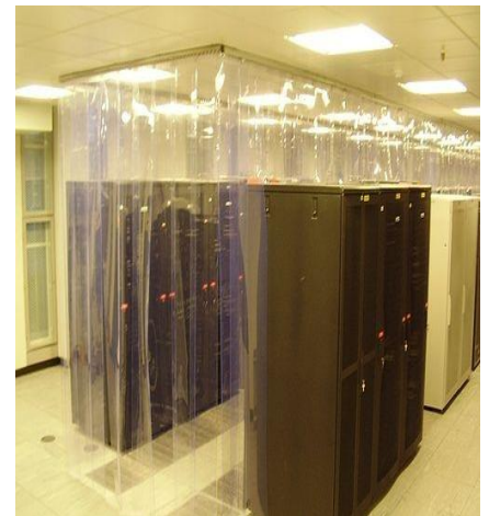
Figure 3: Cold Aisle Containment using vinyl strips
